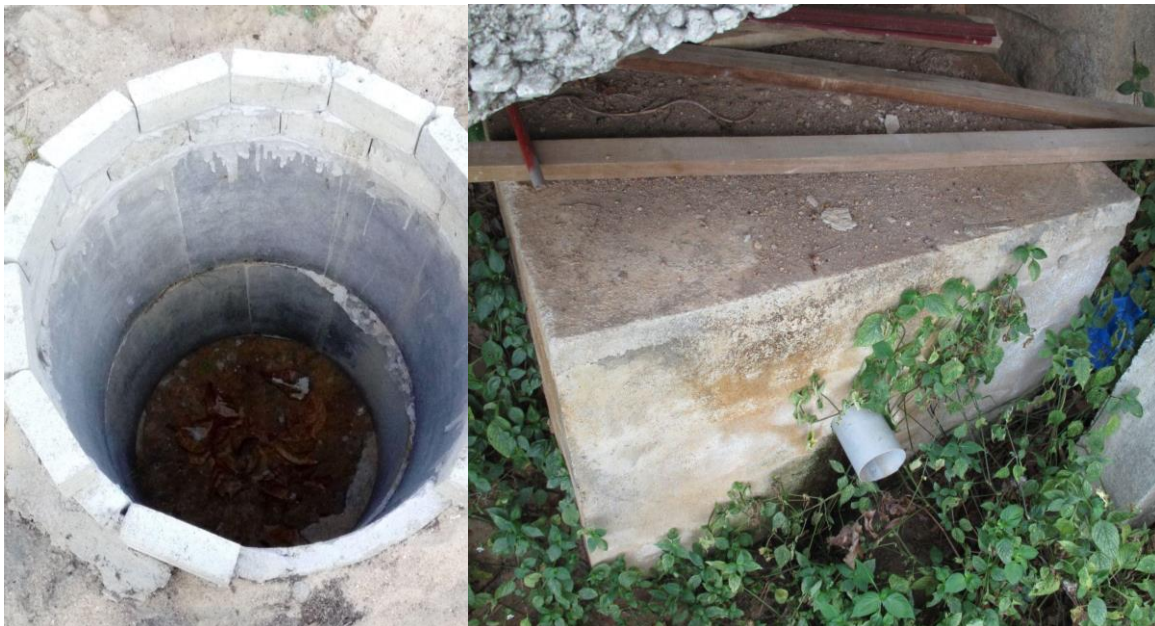
Basic wastewater collection system on Tioman island (Alvin Chelliah, Reef Check Malaysia)
